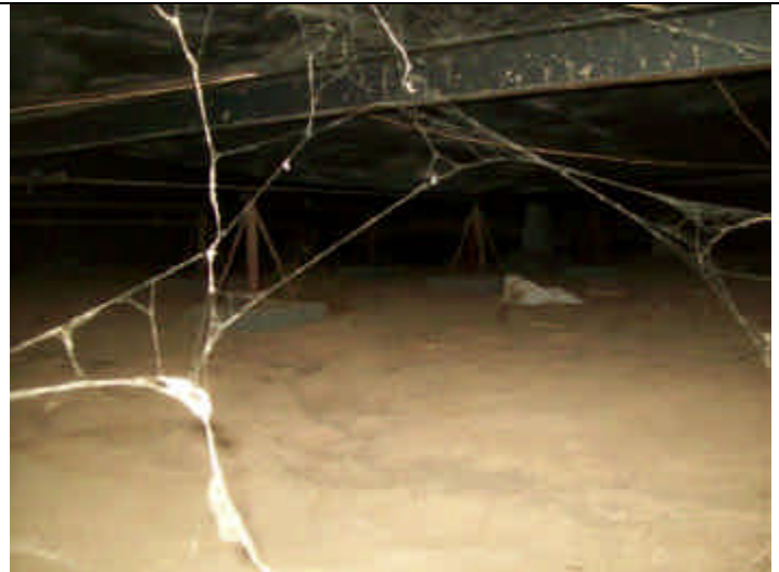
Photo 10: Crawl space view showing masonry & metal piers on concrete pads and perimeter retaining wall.
