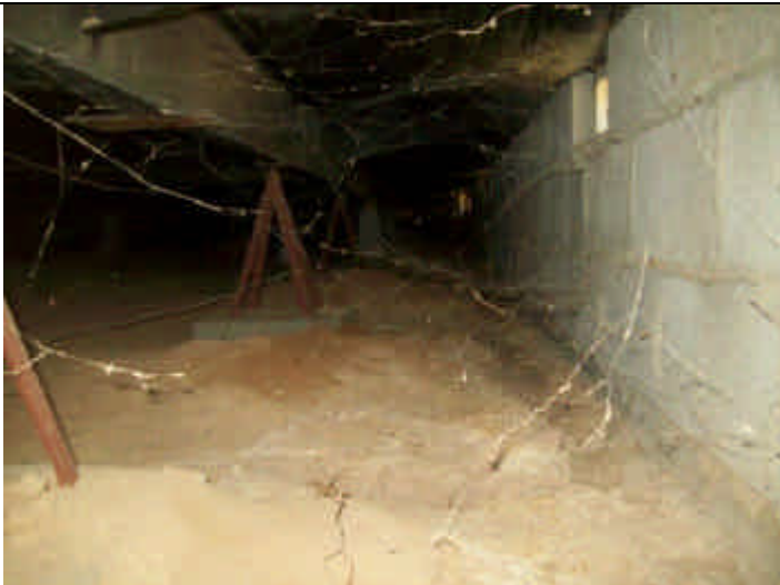
Photo 9: Crawl space view showing masonry & metal piers on concrete pads and perimeter retaining wall.
