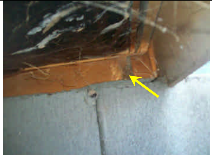
Photo 8: Crawl space view showing metal straps from stem wall and tied to exterior wall.
