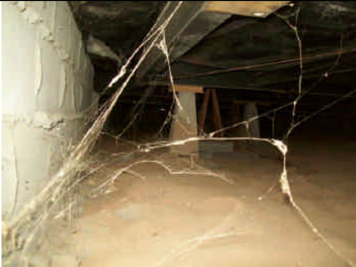
Photo 11: Crawl space view showing masonry & metal piers on concrete pads and perimeter retaining wall.
