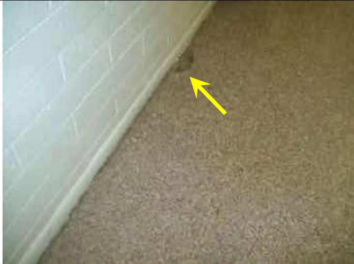
Photo 67: Gaps and tile flooring damaged along south edge of social hall in classroom building.
