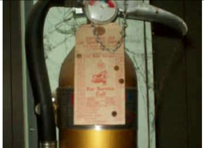
Photo 104: Old fire extinguisher whose certification is over due.
