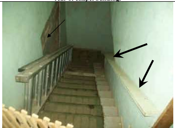
Photo 102: No 'graspable' rail for stairway to basement area in chapel building.
