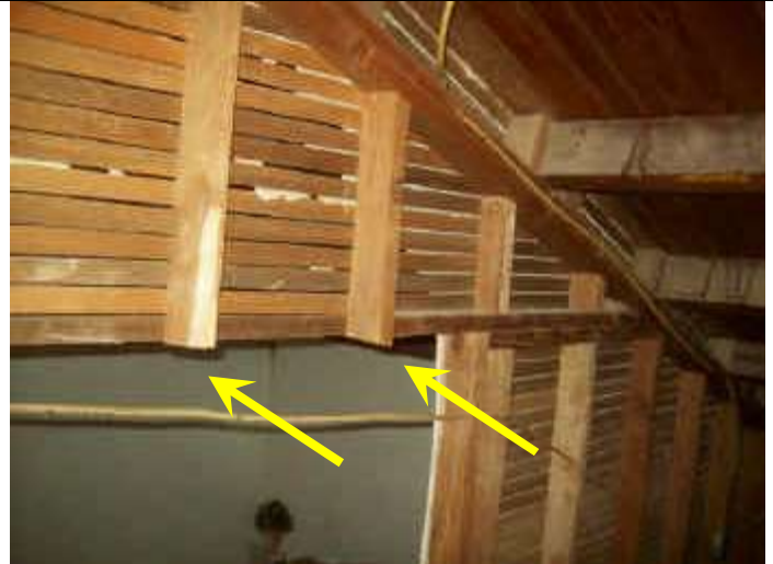
Photo 98: Wall vertical supports cut for HVAC installation, however not subsequently supported.
