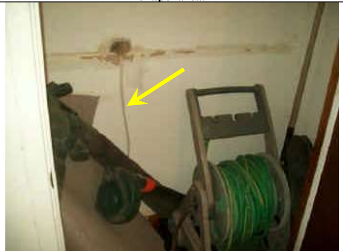
Photo 84: Exposed Romex wiring in storage room at rear or west end of chapel area.
