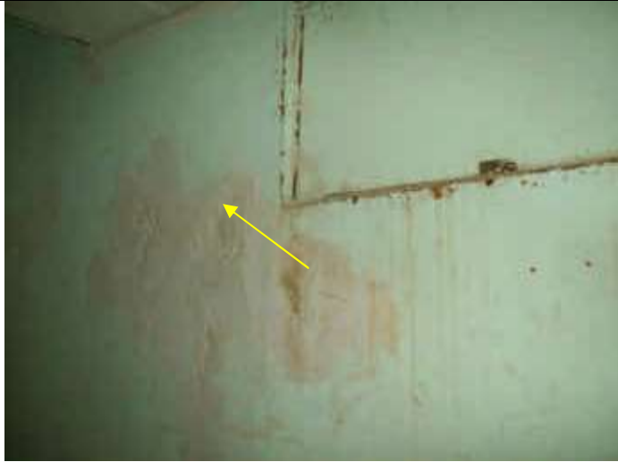
Photo 115: Water stains on interior walls of basement area.
