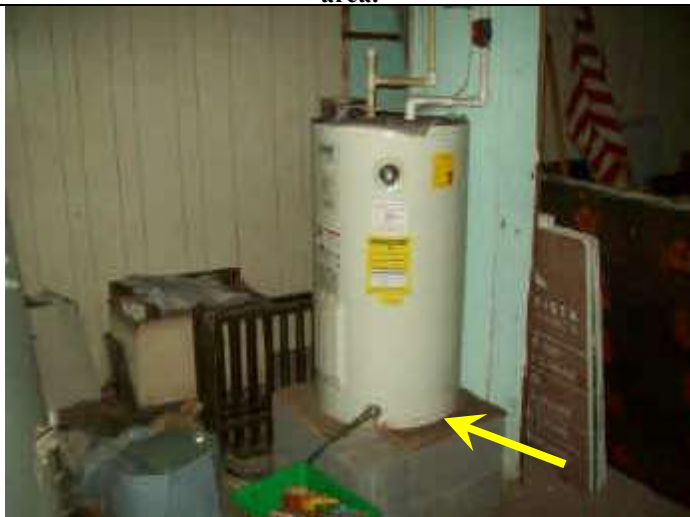
Photo 111: Electric water heater installation in basement of chapel, old unit. With signs of rusting.
