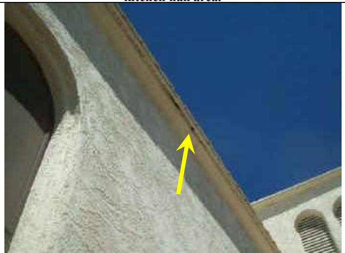
Photo 70: Seams at bottom edges of chapel metal roof separated along south edge, typical.
