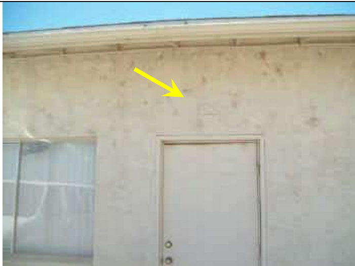
Photo 13: Distress cracks in masonry joints on north exterior wall over door.
