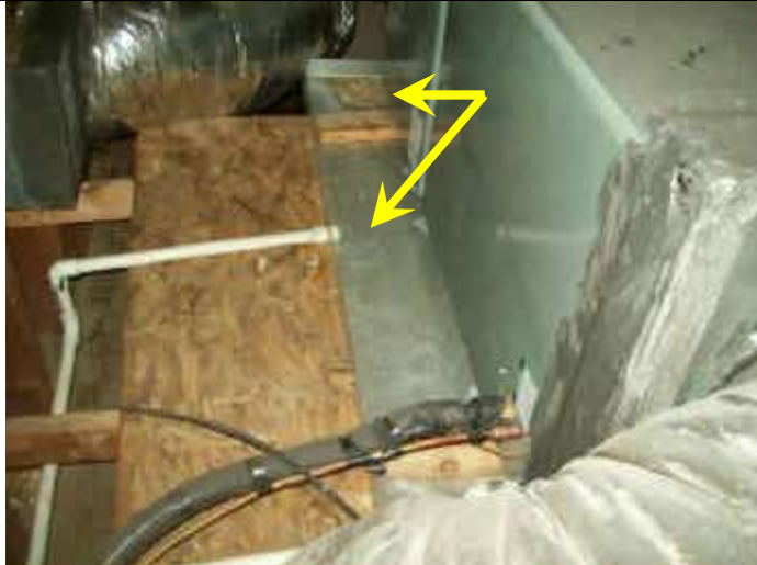
Photo 97: HVAC condensation pan not angled to drain and unit installed on wood blocks in pan for chapel.
