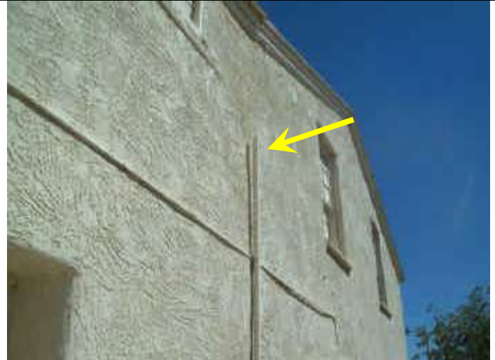
Photo 70: Sewer plumbing line ends along rear wall of chapel and does not extend up past roof line.
