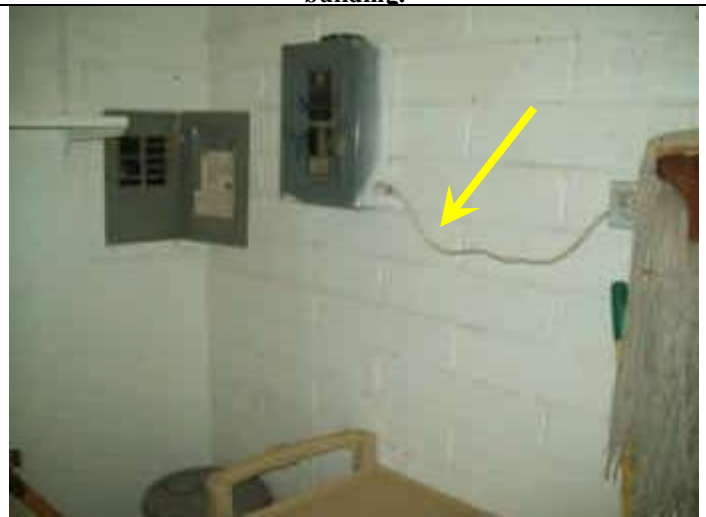
Photo 64: Exposed Romex wiring in storage area by kitchen in classroom building. .
