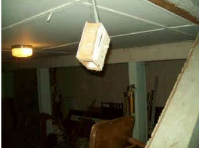
Photo 103: Loose switch outlet at entrance to basement area.
