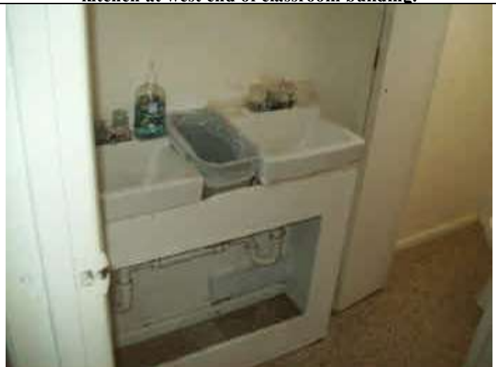
Photo 58: View of sinks in common restroom for kitchen and social hall areas, not ADA compliant.
