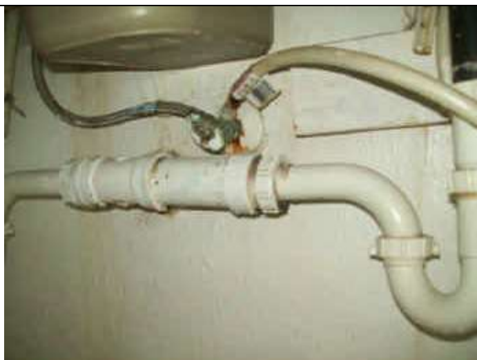
Photo 59: Signs of rusting and previous water leaks under sinks in kitchen hallway area.
