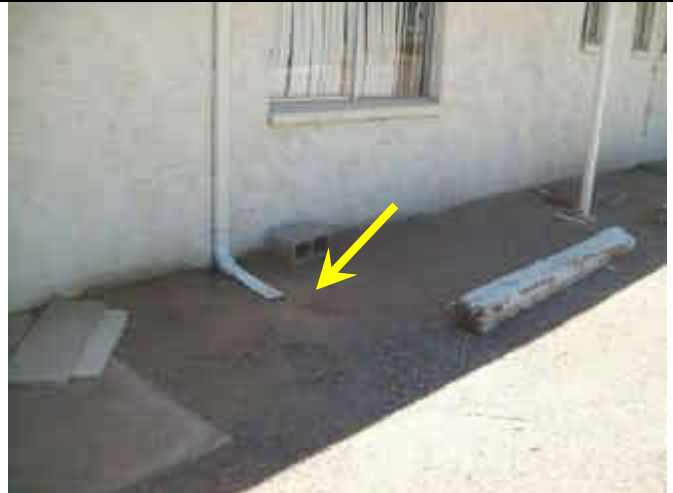
Photo 12: Downspout flattened along north edge of classroom building.
