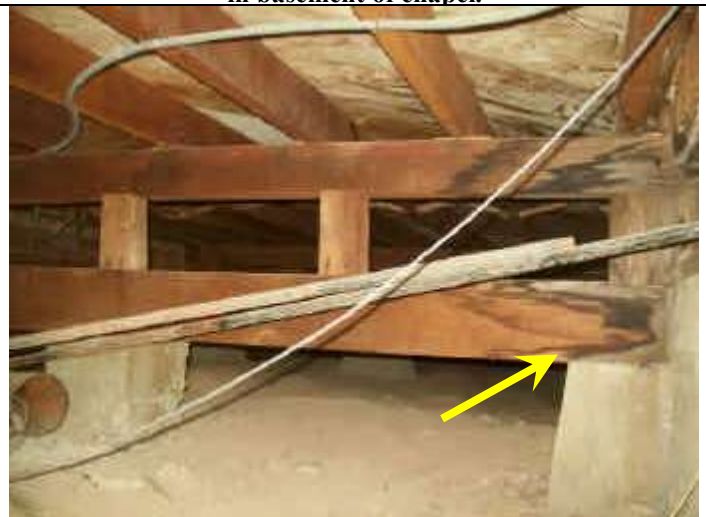
Photo 112: Crawl space view under main chapel area. Water stains noted on header supports west end.
