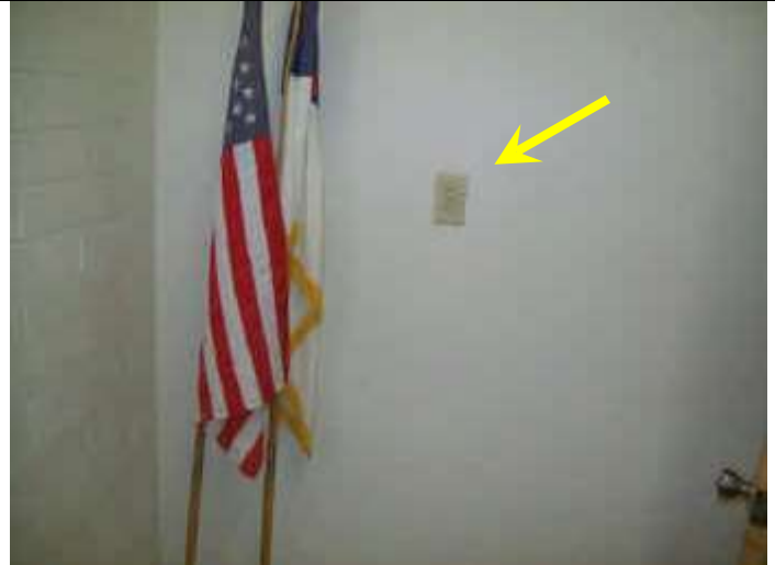
Photo 68: Two-prong outlets noted in storage room of kitchen hall area.
