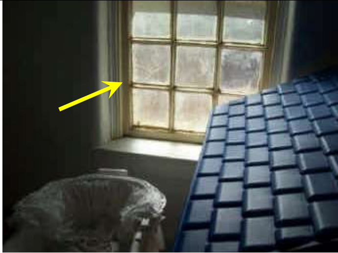
Photo 91: Broken glass panes on rear exterior wood windows.
