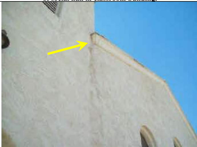
Photo 69: Water drains onto stucco surface along east wall of chapel area. .
