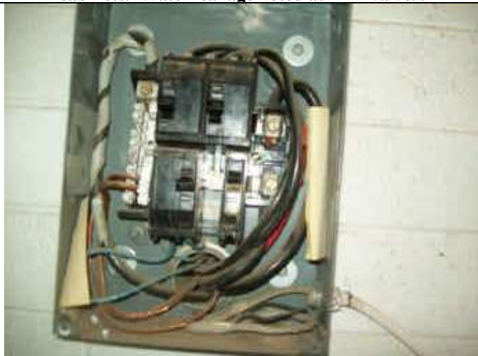
Photo 65: Electrical sub-panel and wiring installation in storage area by kitchen in classroom building. .
