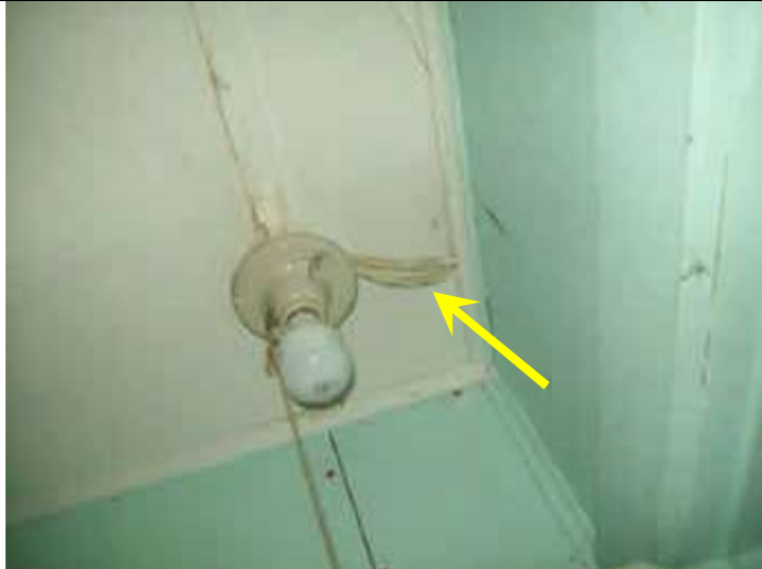
Photo 109: Exposed Romex wiring to switch in basement area.
