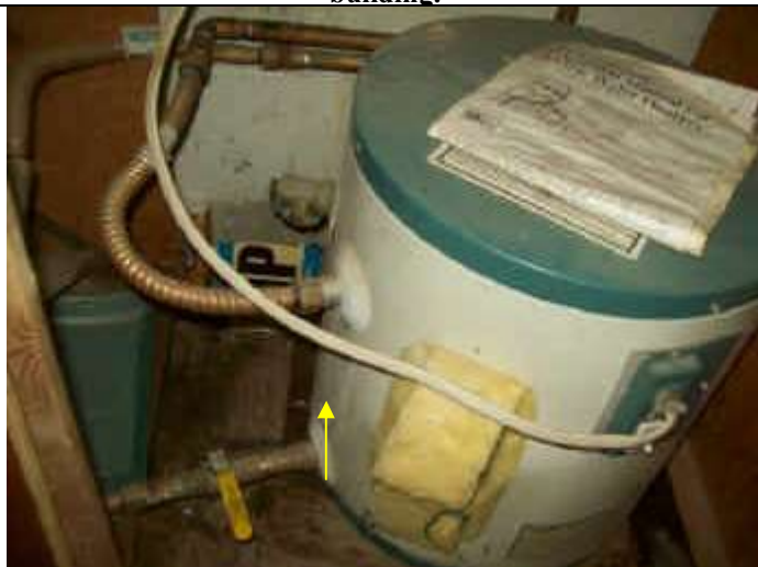
Photo 63: Electric water heater installation in kitchen under cabinets. Water leakage noted at TPR valve. .
