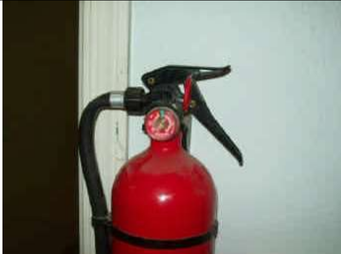
Photo 55: No certification tags on fire hydrants in classroom building areas.
