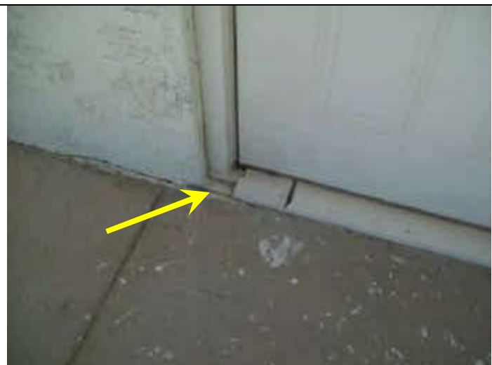
Photo 37: Poor flashing along bottom edge of classroom building exterior doors.
