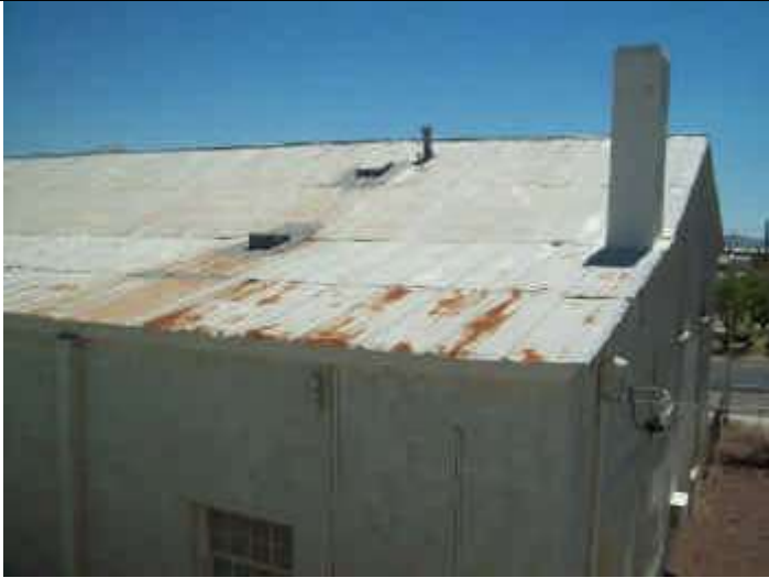
Photo 23: Standing seam metal roof surface view north slope west end of chapel. Rusting noted at bottom edges.
