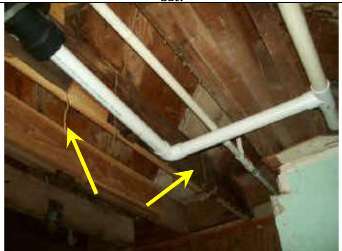
Photo 106: Termite tubes on floor joists along top ceiling area of basement west edge.
