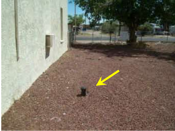
Photo 67: Septic tank clean out along rear exterior of chapel.
