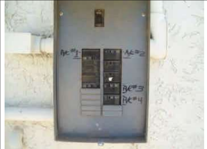
Photo 34: Main electrical service panel on west exterior wall of chapel. Not all breakers labeled. .
