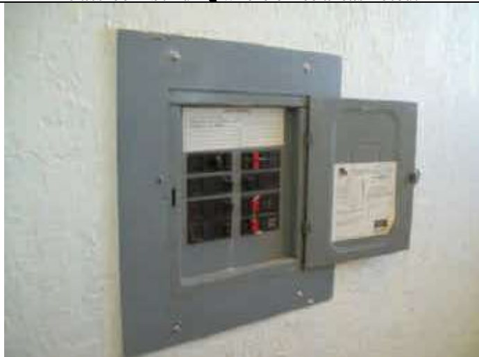
Photo 47: Electrical sub-panel, in east hallway bathroom of classroom building.
