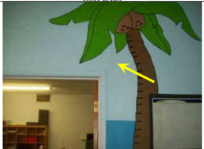
Photo 52: Distress crack on west wall of child care area of classroom building over entry door.
