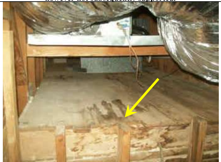
Photo 100: Water stains below HVAC condensation pan at rear of chapel building.
