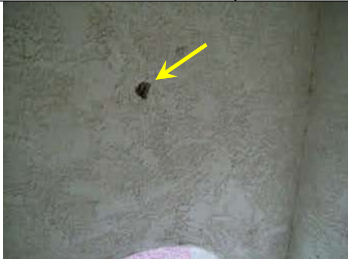
Photo 71: Open electrical junction box on wall above front entry and bell tower area.
