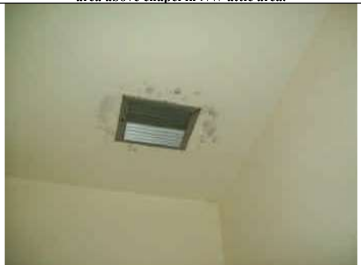
Photo 90: Dark discolorations by air supply register in rear hallway of chapel area.
