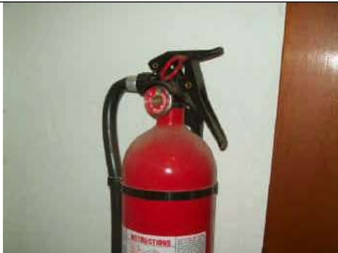
Photo 77: No certification tags for fire hydrants in chapel areas
