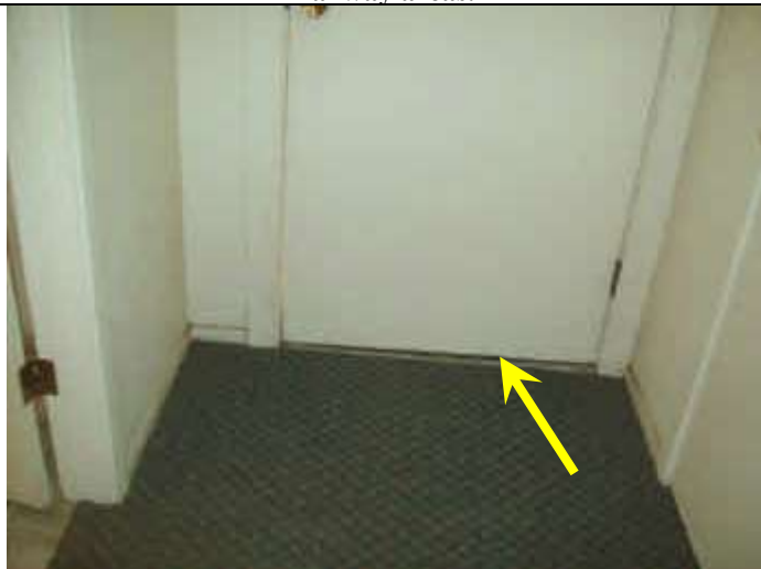
Photo 83: Weather stripping worn around exterior doors of chapel building.
