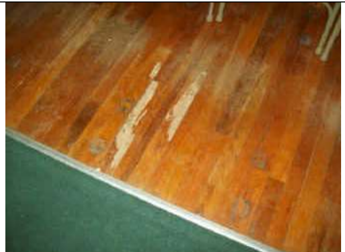
Photo 78: Wood flooring damaged by wood destroying insect activity along east edge.
