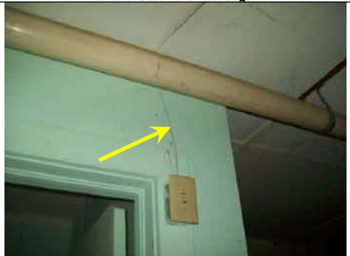
Photo 108: Exposed Romex wiring to switch in basement area.
