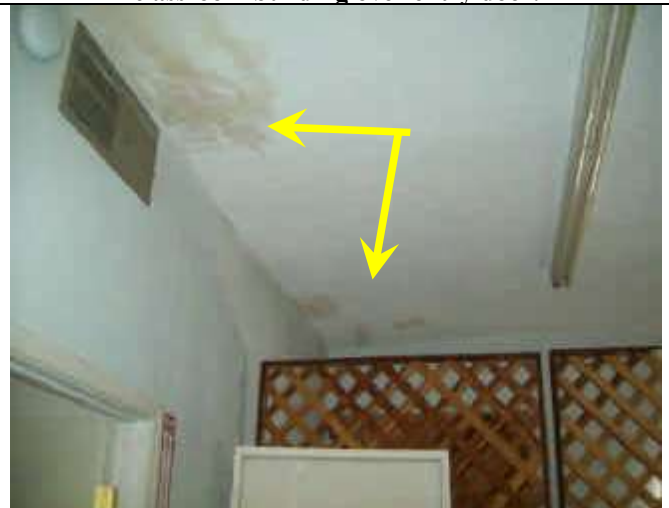
Photo 54: Water stains on ceiling acoustic panels in secondary child care area just east of kitchen area. .
