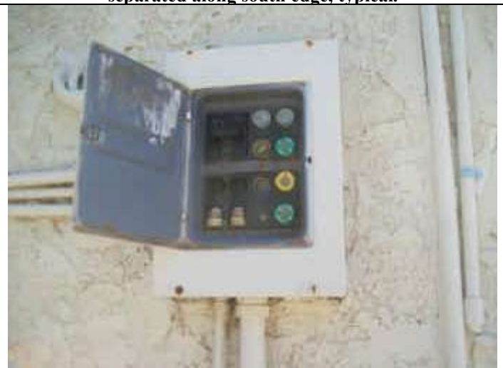
Photo 72: Wiring over-fused in electrical panel on north exterior wall of chapel.
