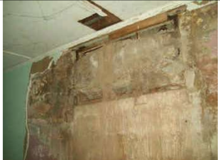
Photo 110: Interior wall surfaces removed at localized areas in basement of chapel.
