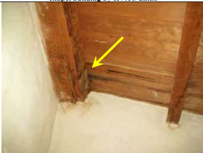
Photo 101: Water stains on wood ceiling area at rear of chapel building south of HVAC installations.
