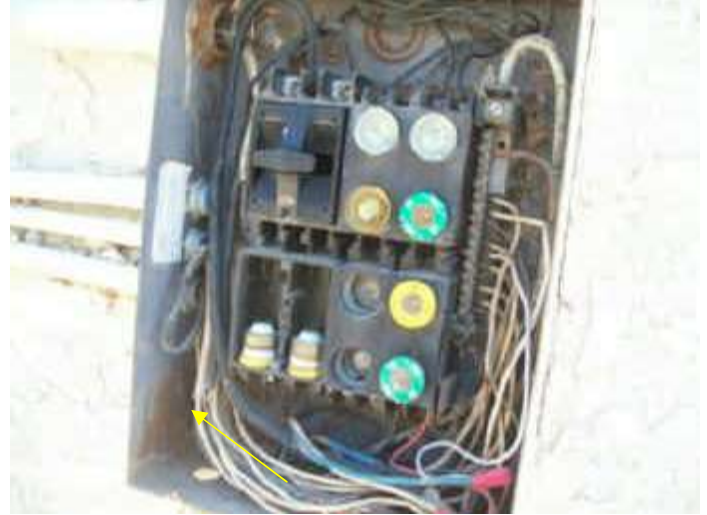
Photo 68: Wiring over-fused in electrical panel on north exterior wall of chapel.
