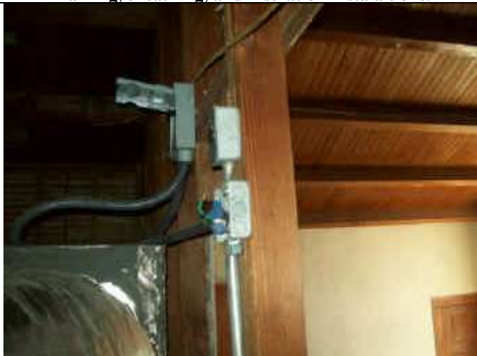
Photo 95: Exposed pigtail wiring at junction boxes at rear of chapel building by HVAC units.
