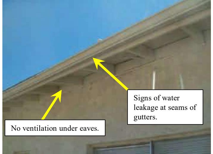
Photo 10: Signs of leaks at gutter seams and no ventilation noted under eaves.
