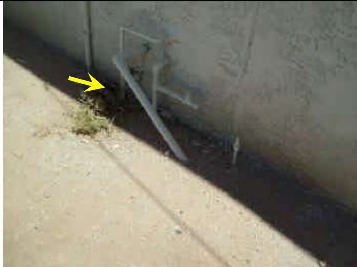
Photo 33: Sewer line comes off north exterior wall of chapel into ground.
