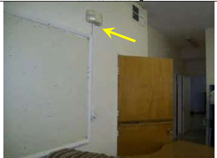
Photo 66: Emergency lighting noted in social hall along north interior wall.
