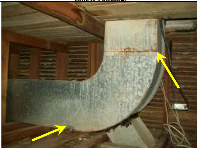
Photo 87: Rusting and signs of water leakage in AC ducting for chapel in NW attic area.
