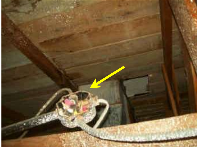
Photo 85: Exposed pigtail wiring in attic area of west end of chapel building.
