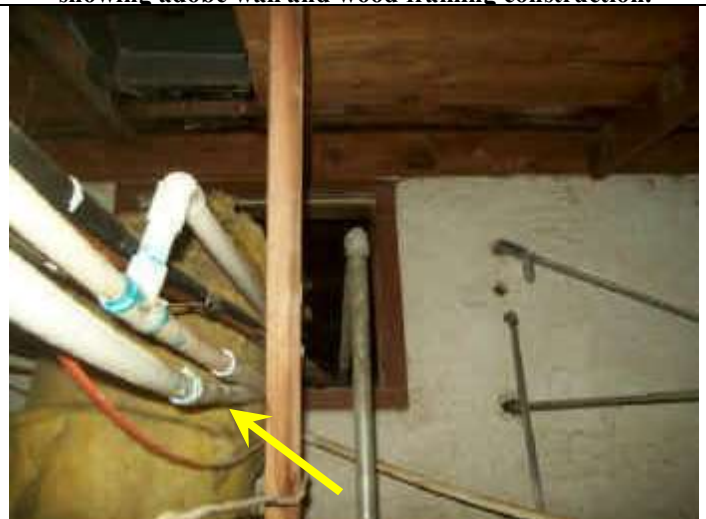
Photo 88: HVAC water condensation line droops in attic area above chapel in NW attic area.
