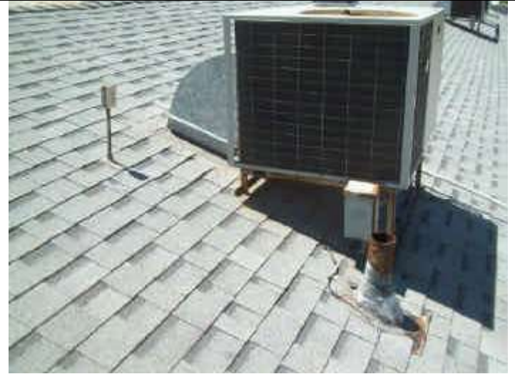
Photo 24: Roof mounted packaged heat pump view on north slope of classroom building roof.
