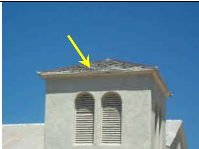
Photo 2: Composition shingle surface worn and deteriorated over chapel bell tower.
