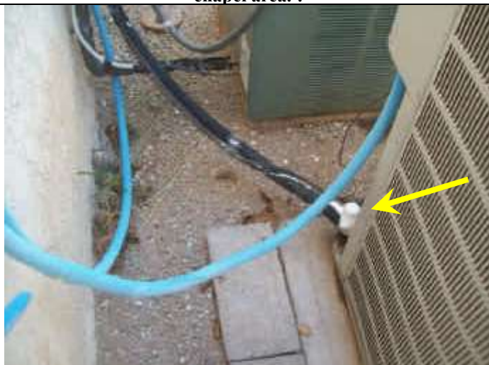
Photo 71: Icing of exterior refrigerant line noted for chapel HVAC compressor/ condenser unit.
