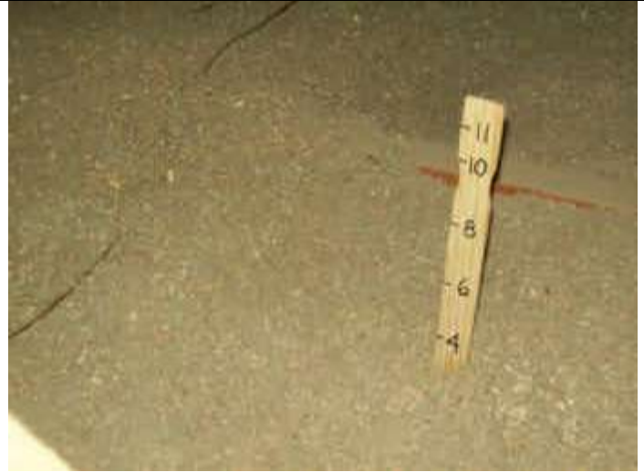
Photo 40: Insulation measured at less than four inches in attic area over classroom building.
