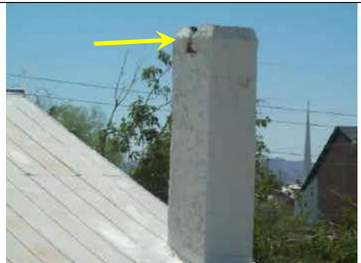
Photo 32: Damage along top edge of chimney stack at west end of chapel building roof.
