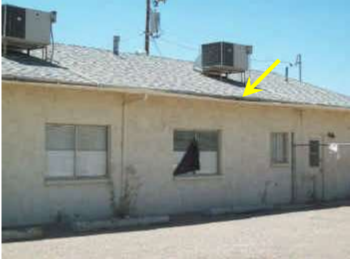
Photo 9: Gutters bent outward along bottom north roof edge of classroom building.
