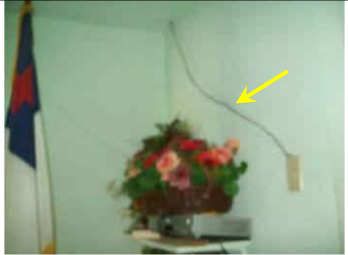
Photo 116: Exposed Romex wiring on interior wall of basement area.
