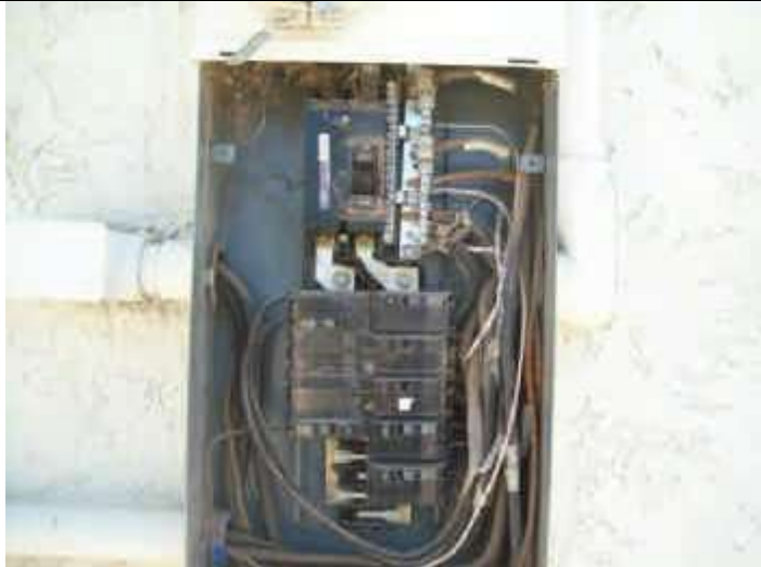
Photo 35: Main electrical service panel and wiring view on west exterior wall of chapel.
