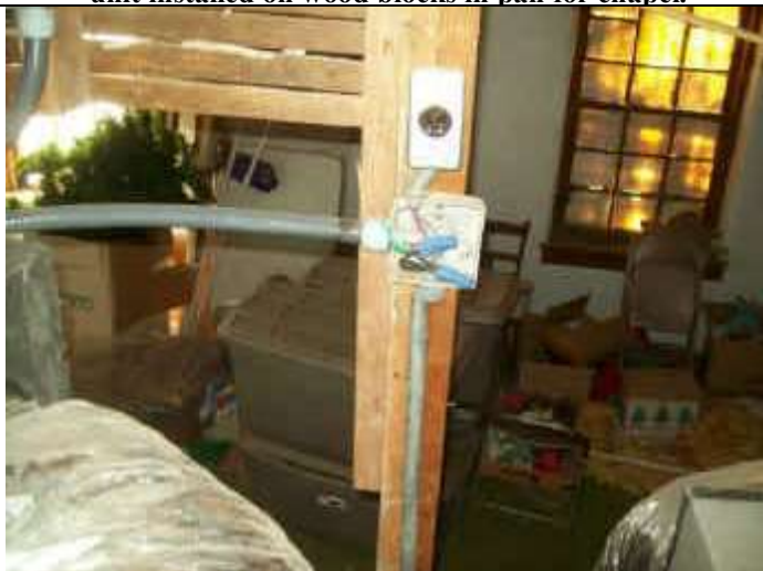
Photo 99: Exposed pigtail wiring at junction boxes at rear of chapel building by HVAC units.
