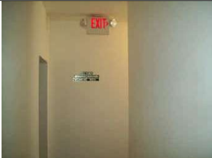
Photo 81: EXIT signage lit and emergency lighting in chapel hallway areas.
