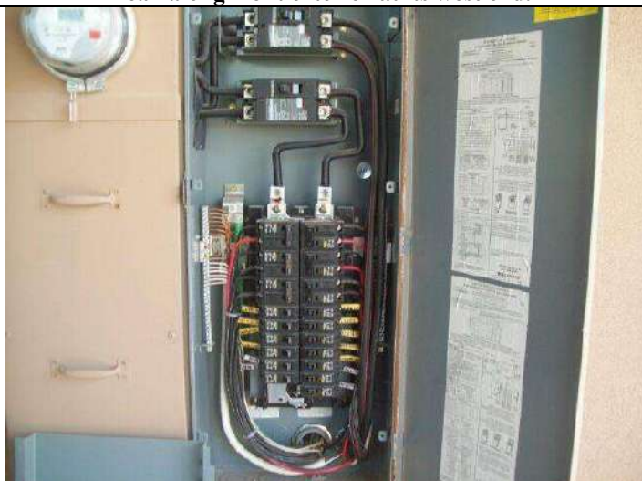
Photo 17: Main electrical service panel and wiring view.
