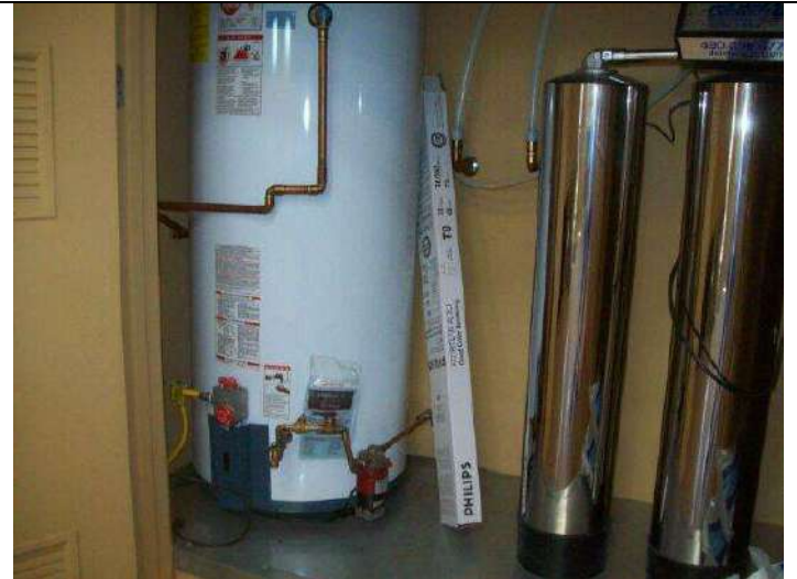
Photo 26: Gas water heater and water softener installation in work room closet area.
