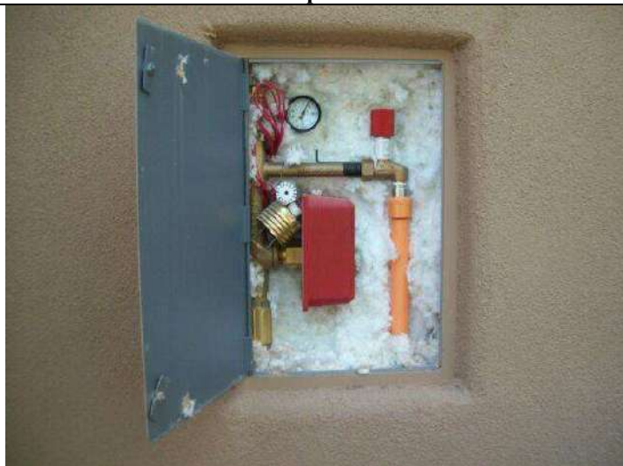
Photo 5: Fire sprinkler system view east exterior wall.
