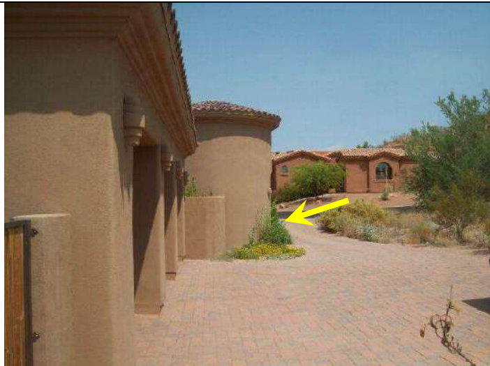
Photo 3: Rear exterior view east end. No access for water to drain and low spot at NE corner.
