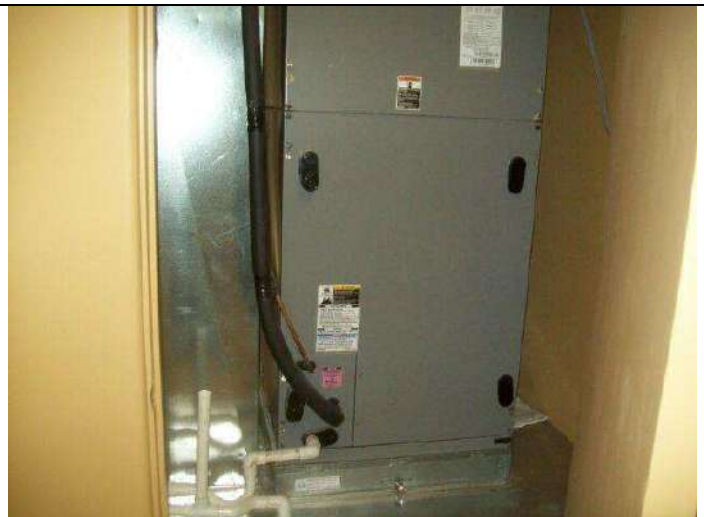
Photo 42: HVAC air handler/ evaporative coil unit in closet area
