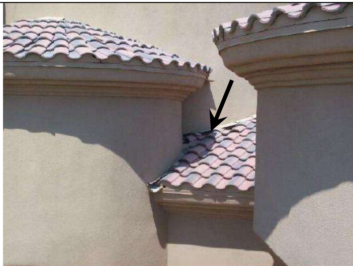
Photo 19: Slipped roof tiles above and east of front entry.
