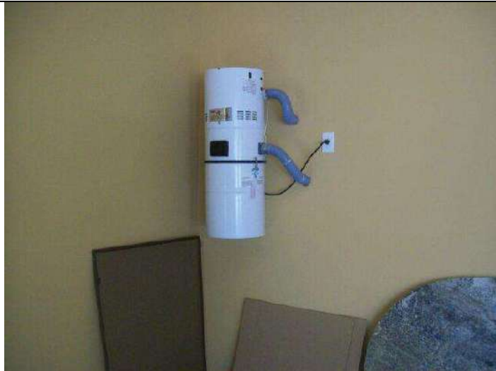
Photo 25: Vacuum system view on garage interior wall.
