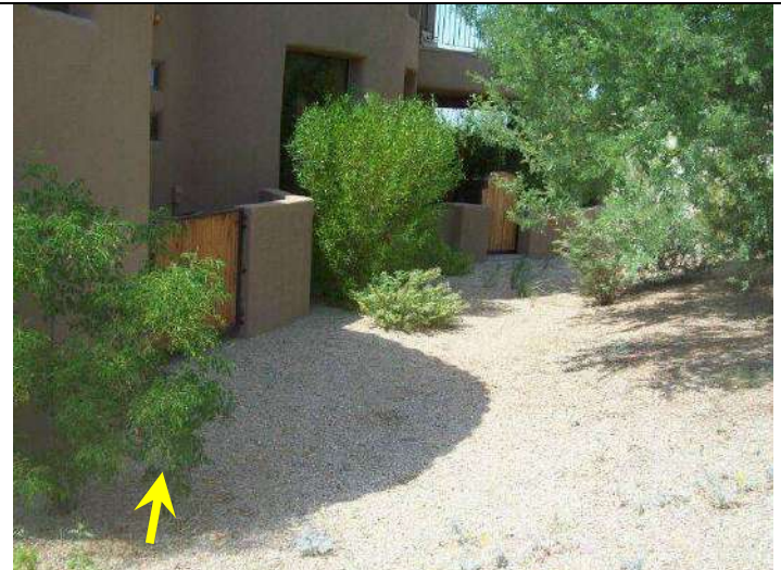
Photo 4: Low spot at NE corner of home. Water flow intended to flow west to natural wash.
