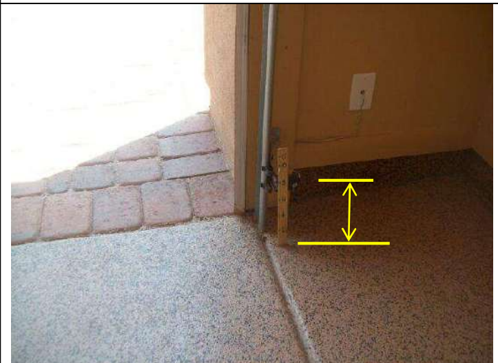
Photo 12: Electronic eyes installed at too high a level at two southernmost garage doors.
