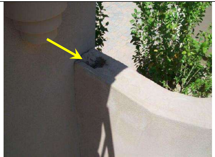
Photo 20: Top of front entry masonry wall not filled.
