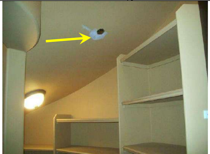
Photo 40: Patch not painted in kitchen pantry area.
