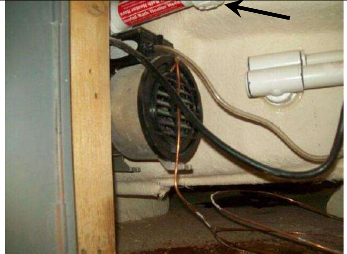
Photo 44: Water leak in plumbing joint for MBR bathroom Jacuzzi tub pump.
