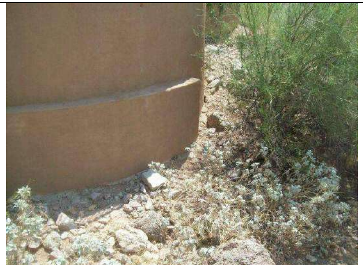
Photo 22: View of drainage along west edge of home. Minor erosion along base of masonry wall.
