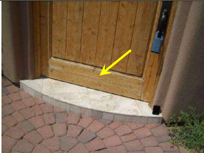
Photo 7: Stain wear on front entry door surface.
