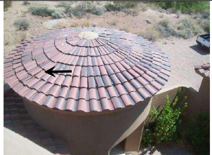
Photo 32: Slipped and unsecured tiles on round tower tile surface and typical of these areas.
