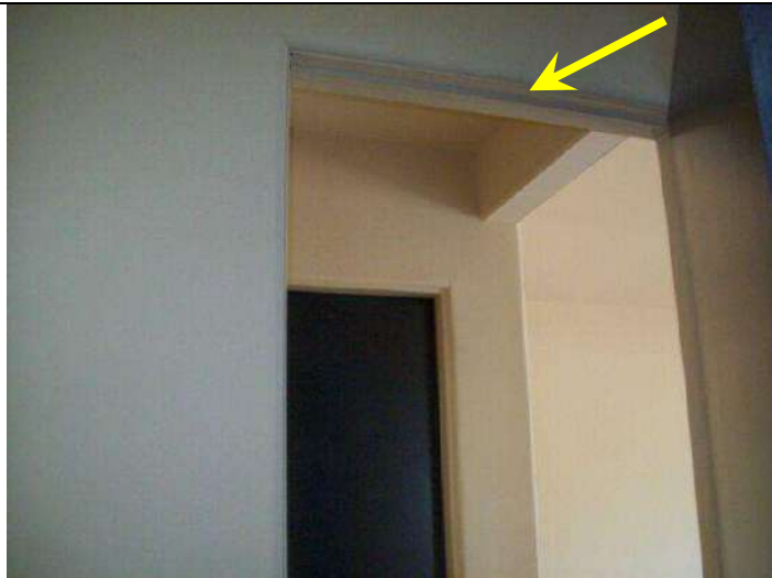
Photo 27: No weather stripping on entry door to conditioned work room off garage area.
