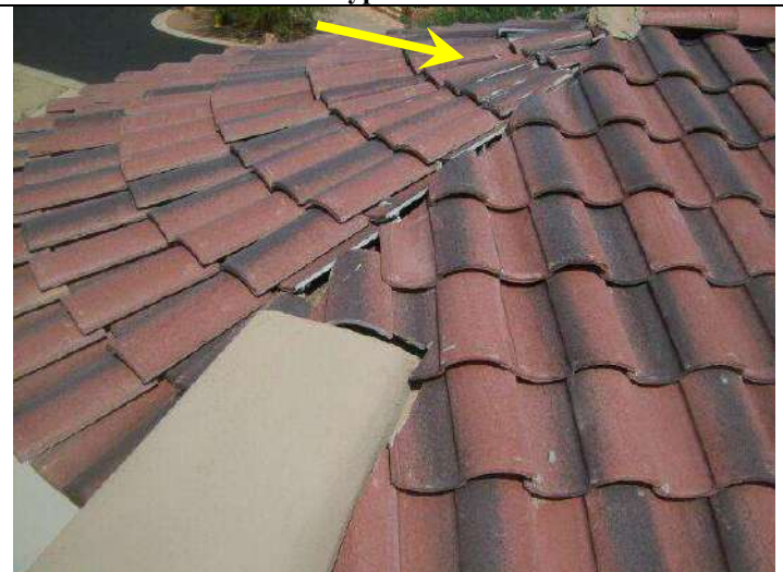
Photo 36: Slipped and unsecured tiles on round tower tile surface and typical of these areas.
