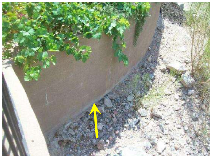
Photo 16: No weep holes noted at base of west masonry wall at its north end.
