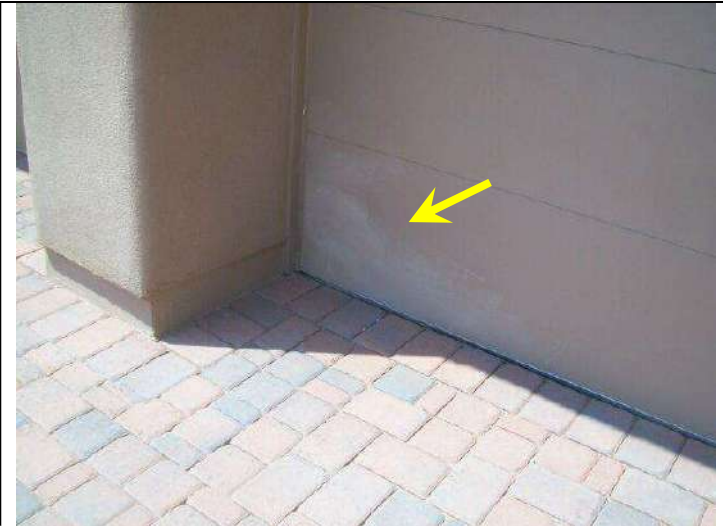
Photo 8: Paint mismatch on exterior surface of garage door.
