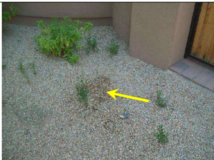
Photo 15: Signs of potential underground sprinkler system leak along front exterior at its west end.
