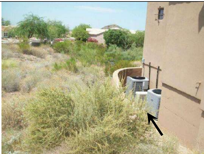
Photo 11: No access for water to drain from rear HVAC installation area.
