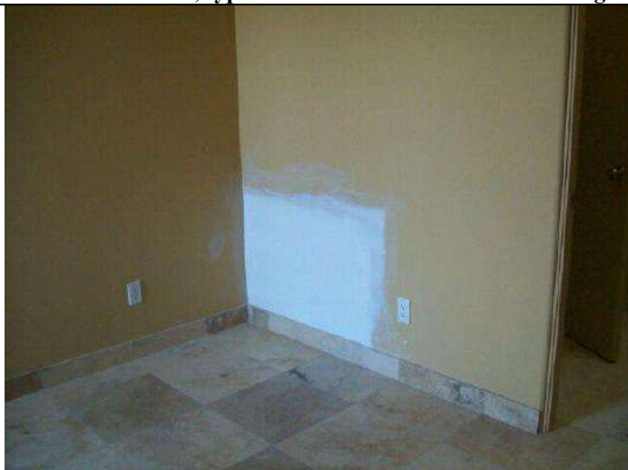
Photo 41: Patch not painted in lower level bedroom.
