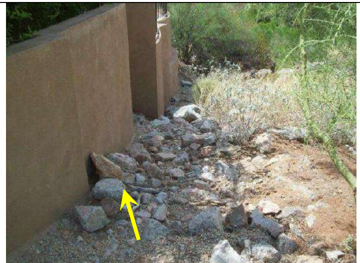
Photo 6: View of drainage along west edge of home. Minor erosion along base of masonry wall.
