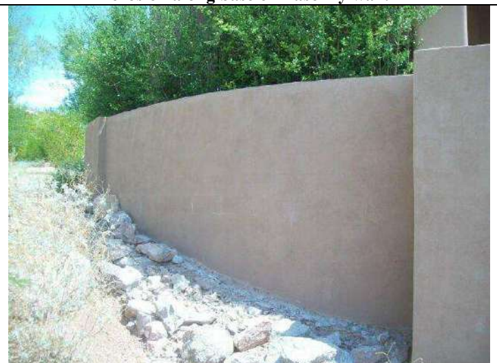
Photo 24: View of drainage along west edge of home. Minor erosion along base of masonry wall.
