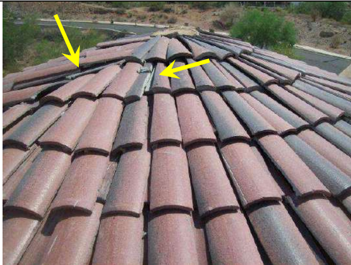
Photo 37: Slipped and unsecured tiles on round tower tile surface and typical of these areas.
