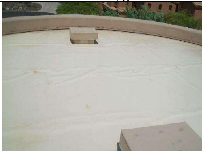
Photo 35: Buckling of rubber membrane surface at NW corner of home.
