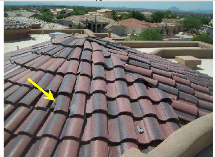
Photo 34: Slipped and unsecured tiles on round tower tile surface and typical of these areas.
